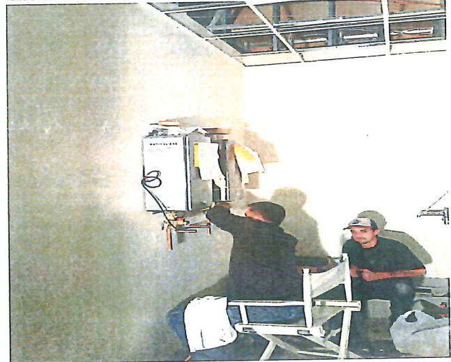
Electrical Panel View 04/04/2013
