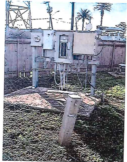
Control and electrical panel board Electricity access
