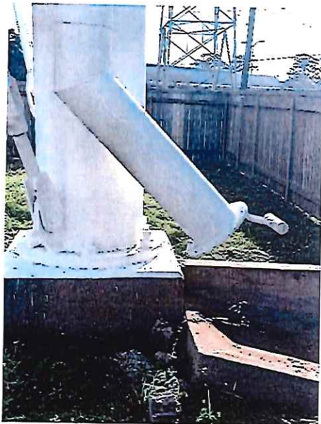
Overflow Pipe – good condition Mildew
