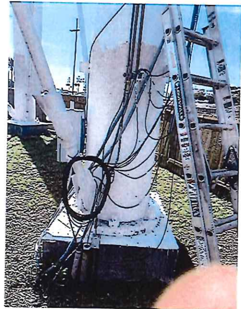
Excess coax to be removed and fastened to the ladder
