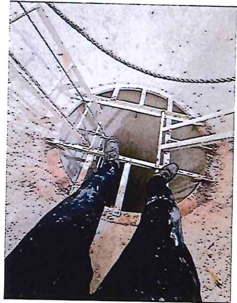
Riser Railing – good condition Rusting and paint failure
