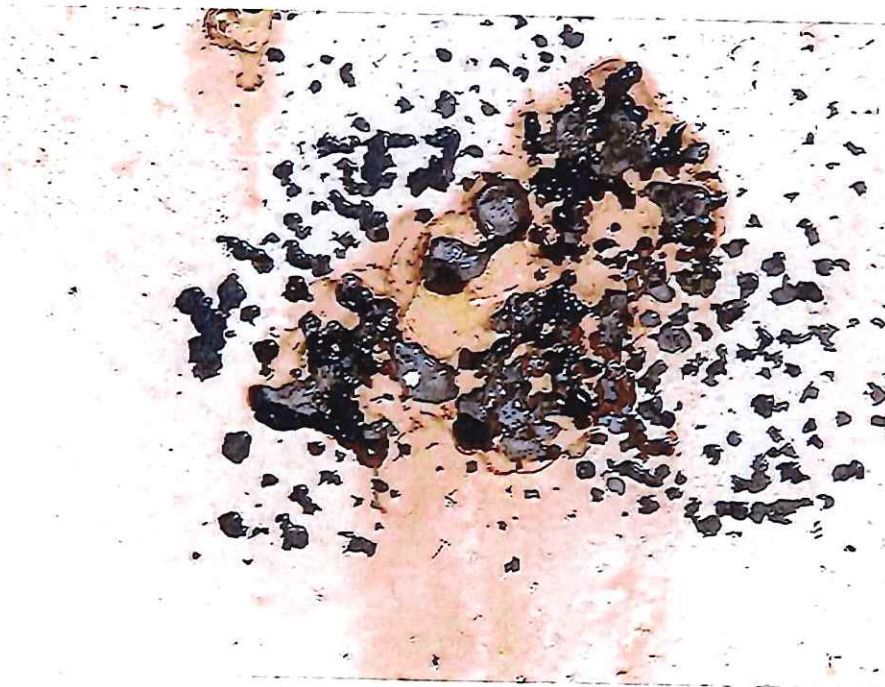
Interior Floor – Severe Pitting, paint failure and rusting
