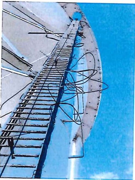
Hanging/tangled coax on the access ladder
