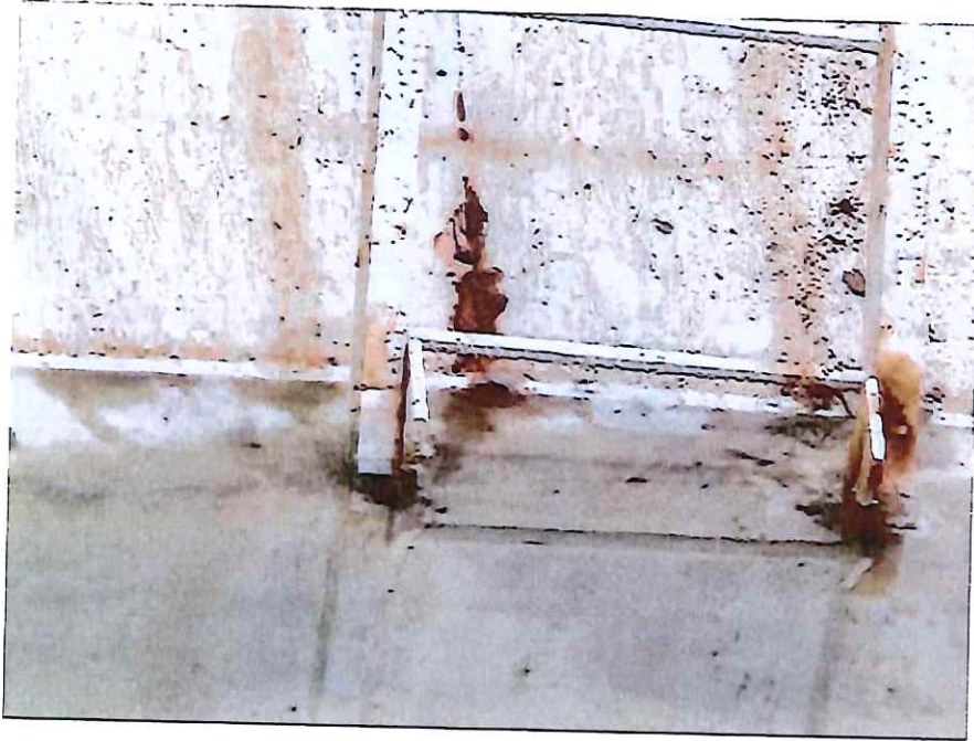
Interior walls – pitting, rusting, chalking, paint failure
